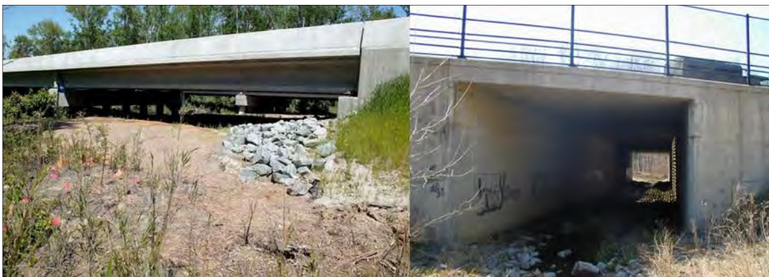
Figure 2. Bridge Underpass Beneath U.S. Highway 17 (left); Large Box Culvert Beneath Fairfax County Parkway (right). Both are used frequently by deer and other wildlife (Donaldson, 2007; Donaldson and Schaus, 2009).
