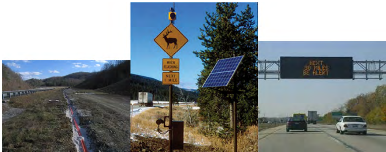
Figure 1. Driver Warning Systems. Buried cable animal detection system during installation ( left ); flashing warning system that can be connected to a detection system ( center ); dynamic message sign ( right ).
